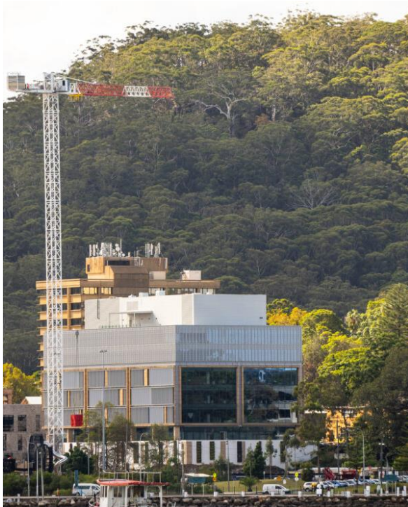
Multi-story buildings under construction on the Central Coast (Credit: Central Coast Council)
