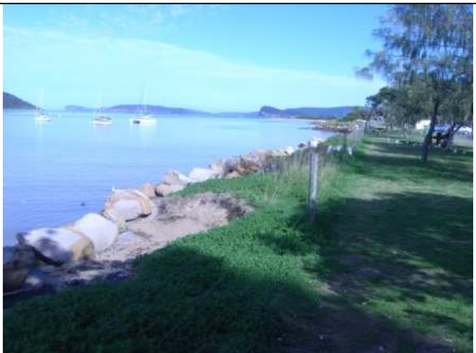
Photo 12: Looking south along Ettalong foreshore – seawall with adjacent recreational area. Lack of beach
