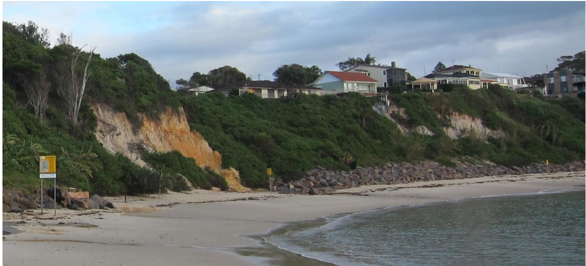
Figure 3-49 Cabbage Tree Harbour Beach and Tall Sand Bluffs looking east, showing the Actively Retreating Indurated Sand Cliff (left) and Toe Protection Structure that Protects the Developed Length of Sand Bluff (middle-right).
