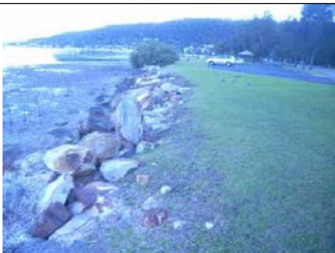
Photo 23: Erosion and rock armour along the Koolewong Foreshore. (W69)
