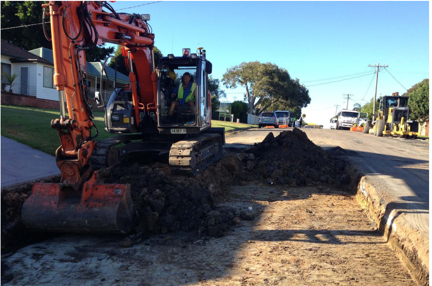
Works continue on upgrading the road and drainage along Lakeside Parade, The Entrance.
