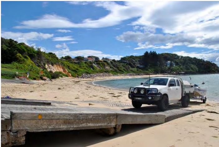
A boat launches off the uneven ramp's surface
