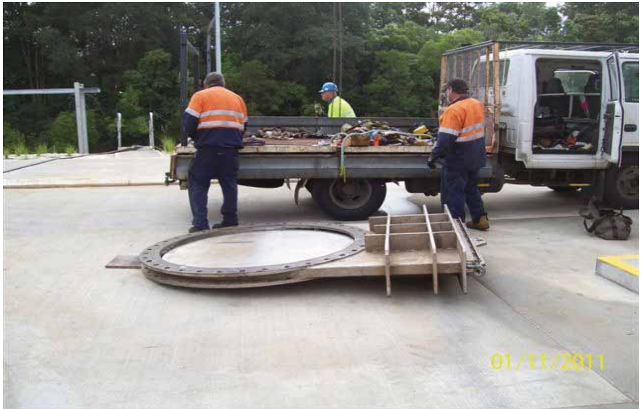
WP 02 knife gate valves prior to installation (Work Package 2)
