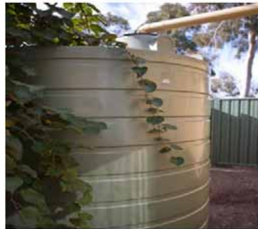
Rainwater tank (M. McAulay & DEWHA).
