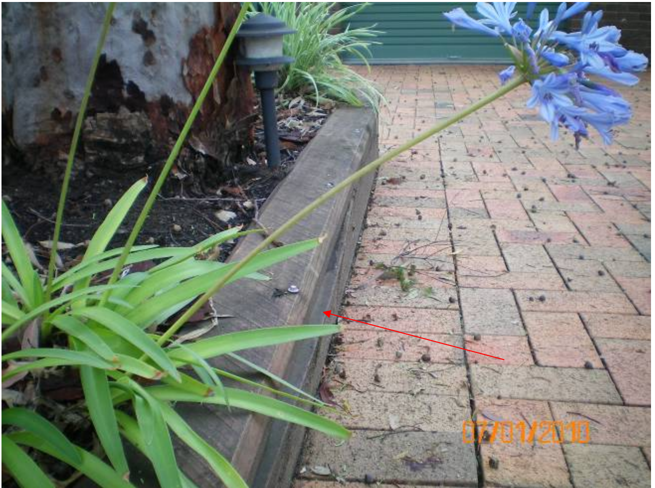
Minor deviation of the retaining wall
