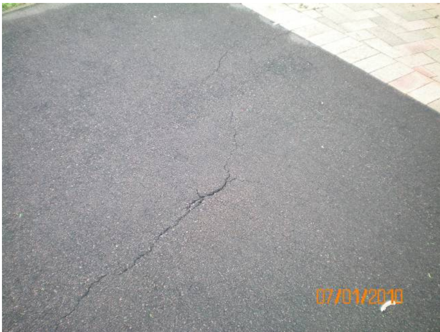
Minor Cracking of bitumen driveway
