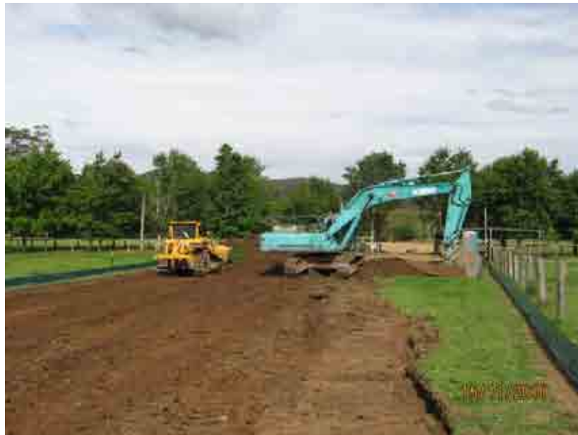
Site preparation of the pipeline corridor (ch 7600) to prevent fertile top soils being contaminated with sub soil material.
