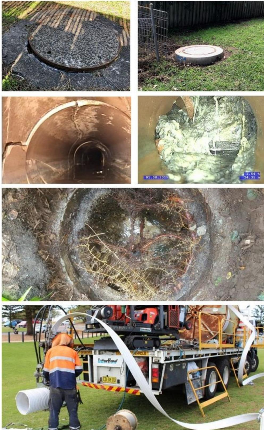
Photo line: 1 broken man hole and repaired and raised manhole from the reveal and seal program, 2 cracked and collapsed sewer pipes which have been fixed, 3 root intrusion, 4 pipe relining.
