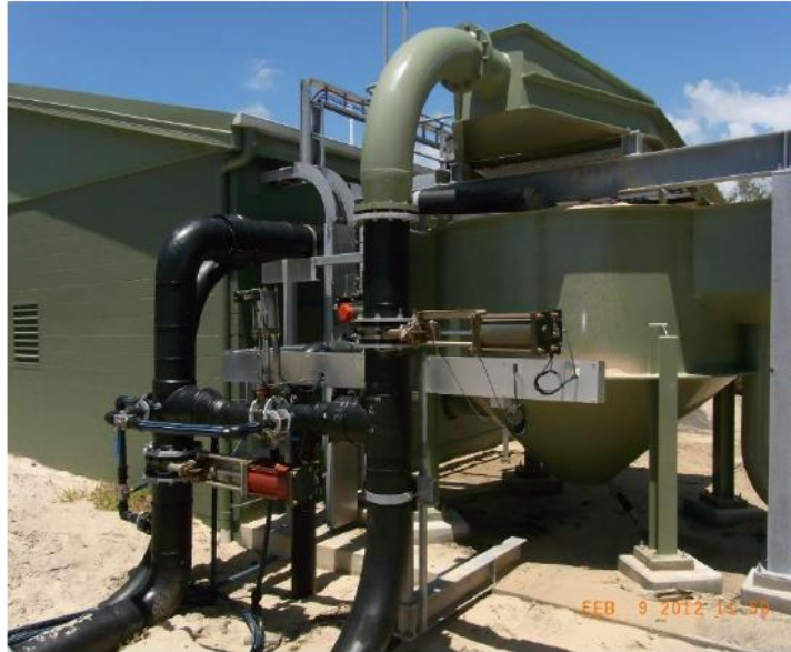
Figure 5-3 Permanent bypass infrastructure at Noosa (courtesy of SCRC)
