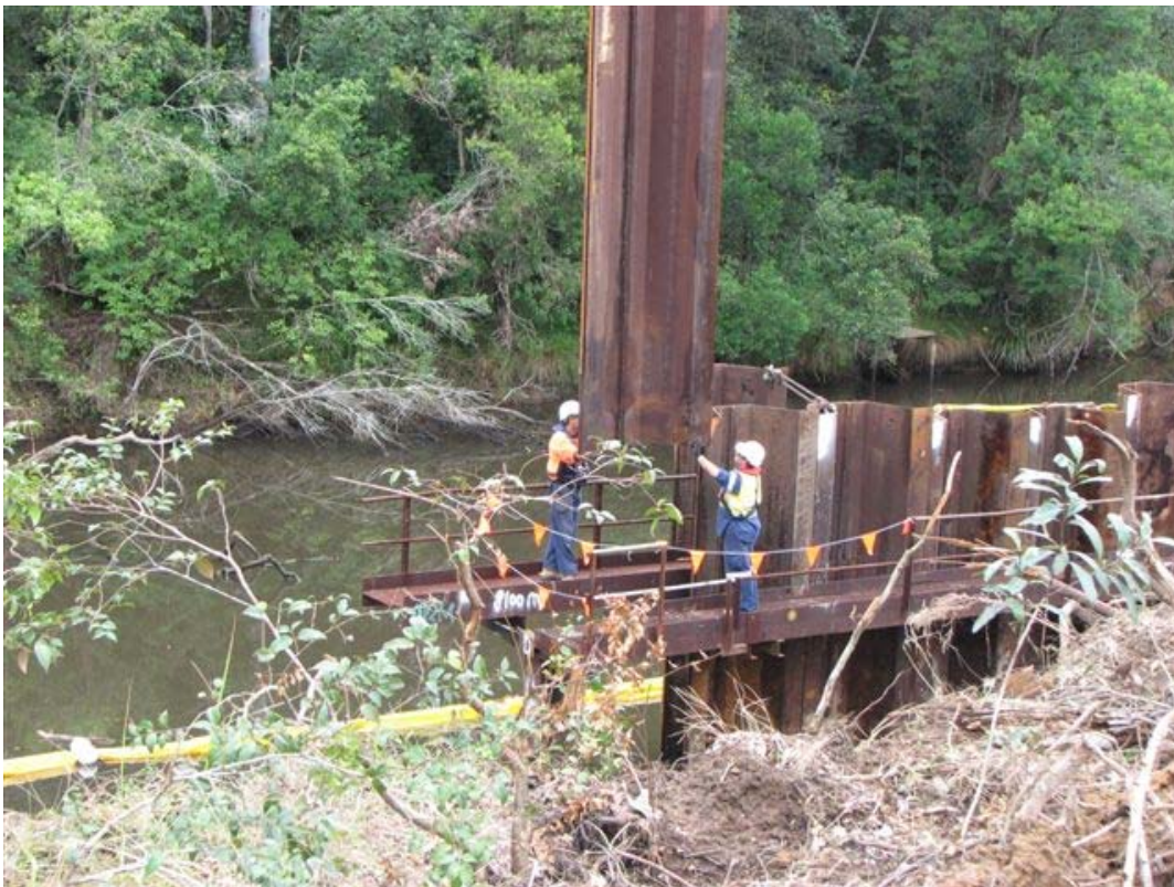
Photo: Sheet piling for coffer dam at Wyong River Off-Take Structure. 16 April 2010.
