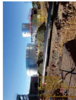
Advanced water treatment plant under construction for the Kooragang Industrial Water Scheme
