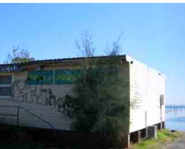
Fig 4.4.4 Upgrade and encourage better use of dilapidated buildings that detract from the ambience and amenity of the Tuggerah Lake Foreshore (Source: Dickson Rothschild)
