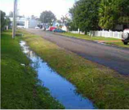
Fig 3.3.1 Lack of Kerb/ Gutter in Long Jetty (Source: Dickson Rothschild)
