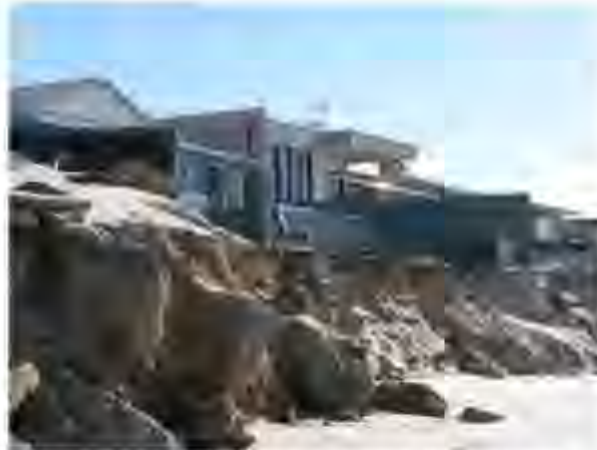
Figure 4.1. Erosion at North Entrance, Wyong Shire (12 June 2009).
