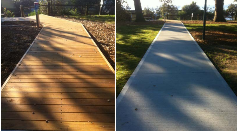
The shared pathway at Toowoan Bay Park joins the new timber boardwalk on The Entrance Coast to Lake Walk
