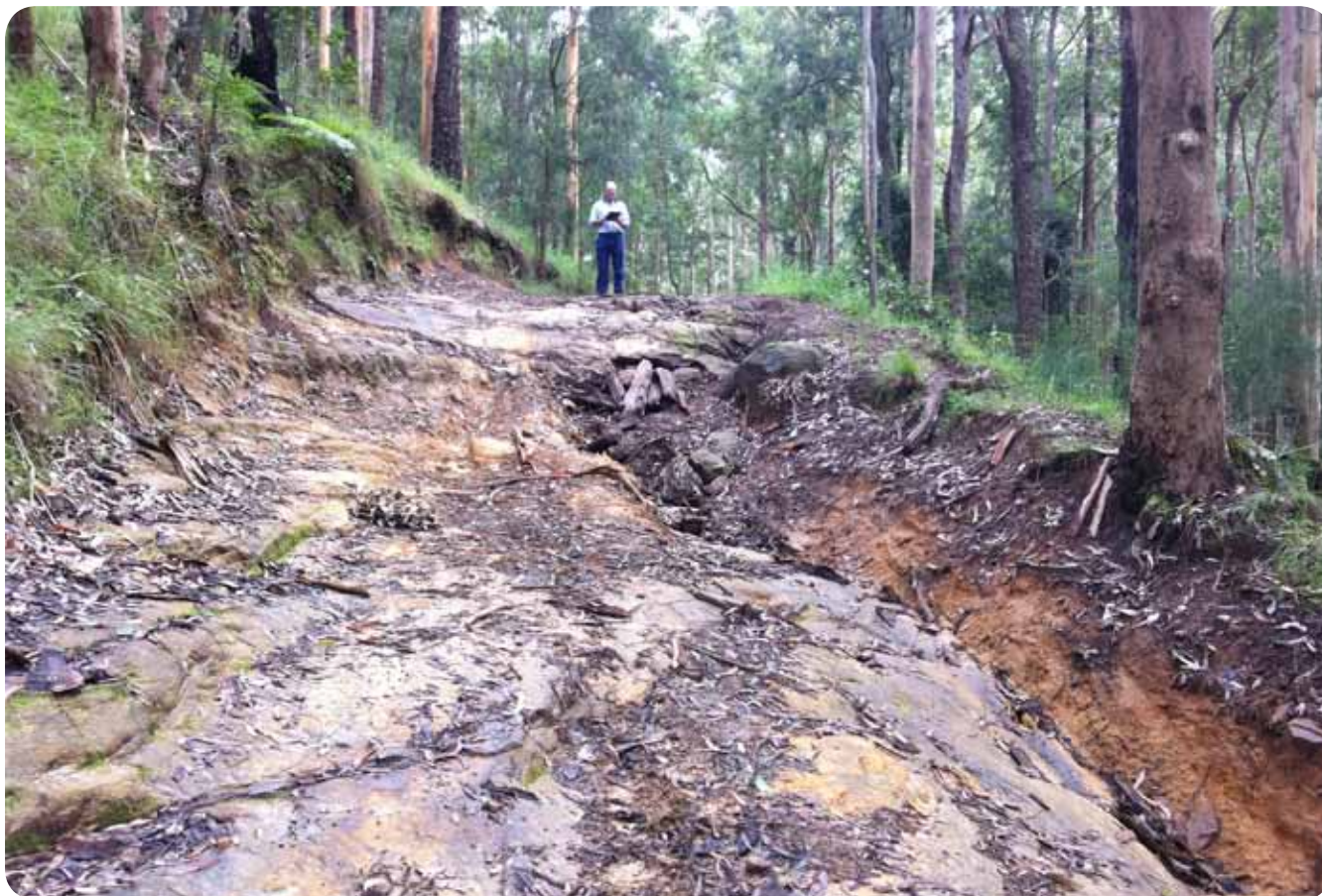
Above the before photo of the fire trail in Dooralong Valley - Opposite the fire trail after $40,000 of work carried out
