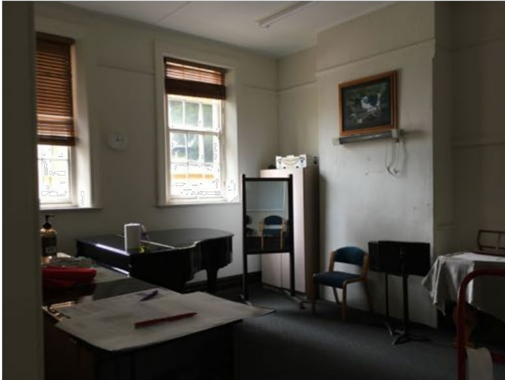
Figure 9: Subject Site: Internal teaching space along the northern boundary. Mould and moisture damage evident.
