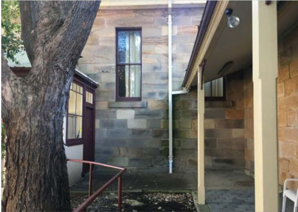
Figure 6: Subject Site: Current Mann Street entry. View of awning to be replaced and new entry and awning incorporated.
