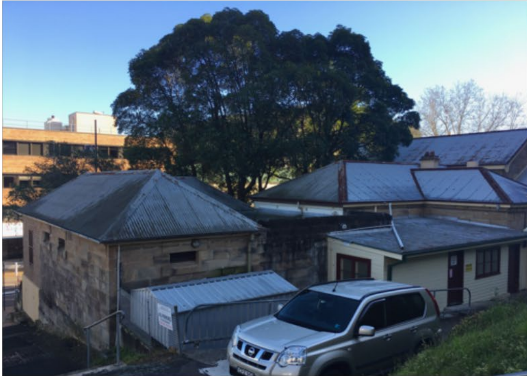
Figure 4: Subject Site. State of existing roof which has been replaced. Also visible add ons to be upgraded.
