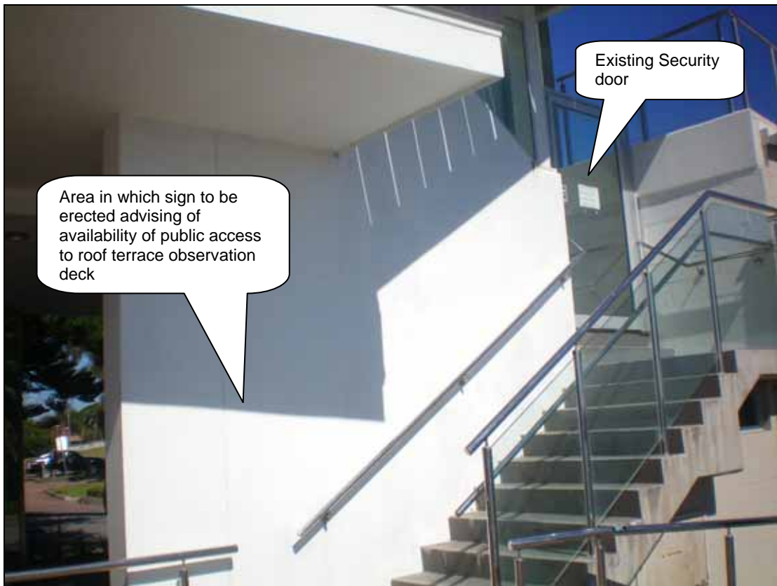
Figure 1: Location of the existing security door installed to the roof terrace observation deck and area that sign is to be erected advising of public availability to the roof terrace observation deck, free of charge.
