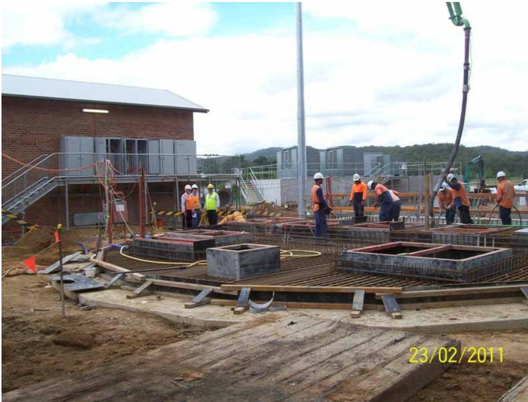
Formed the roof slab of the wet well and poured on 23 February 2011 for the Wyong River Pump Station ( Work Package 2 ).
