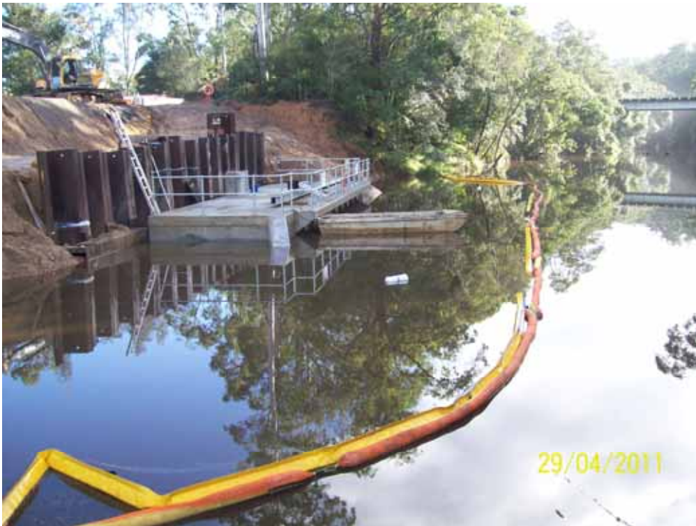
Wyong River Off-take Structure with inlet pipes to Pump Station flooded (Work Package 1)
