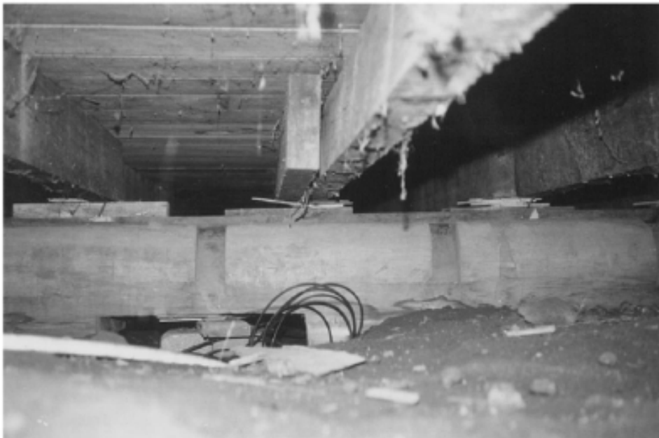
Plate 7: The Homestead in the 1980's indicating the floor has been replaced using modern timber joists and flooring, noting the check-outs in the bearer joist.. (Source - WDM&HS)
