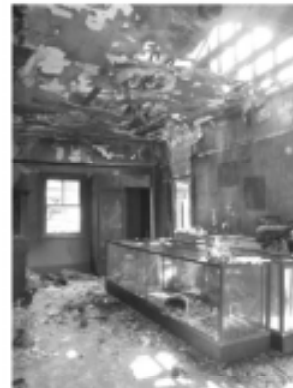
Plate 16: The extensive damage to Room 2, with hardwood framed walls still standing.
