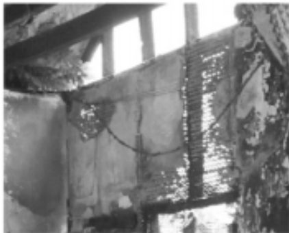
Plate 9: The remains of metal lath used on walls.
