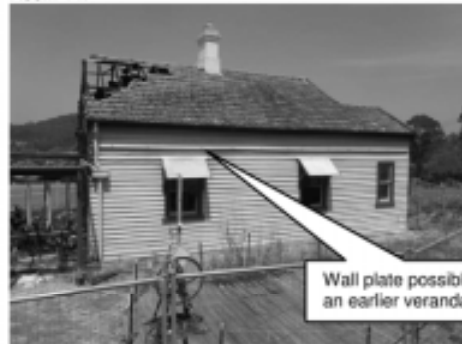
Plate 22: Burnt northern wall to Room 3 from the west.
