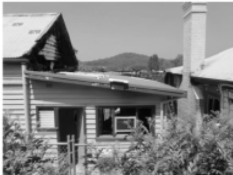
Plate 21: Burnt out gable over Room 14.
