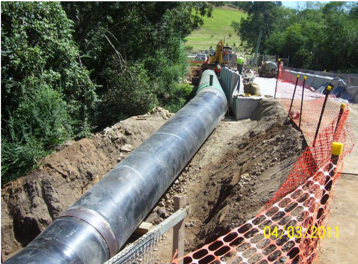
Bunning Creek road bridge with Mardi to Mangrove Transfer main fitted into position. (Work Package 7)
