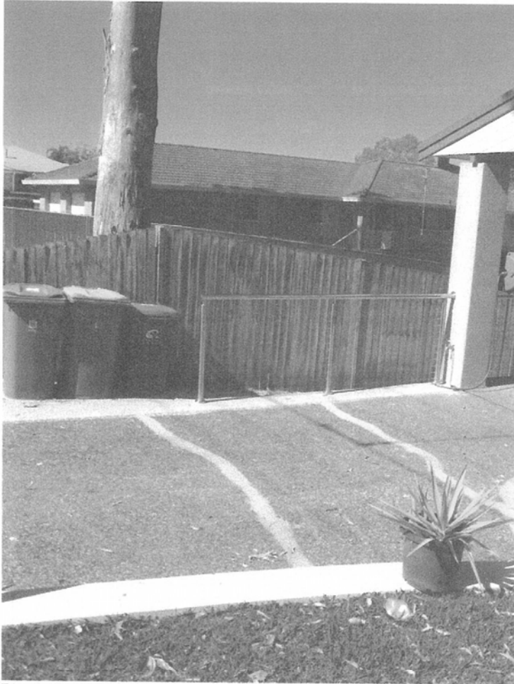
Photo. 3 The trunk of the small fruited grey gum and the driveway of number 60 Gordon Avenue. Please note the damage to the driveway and the boundary fence.
