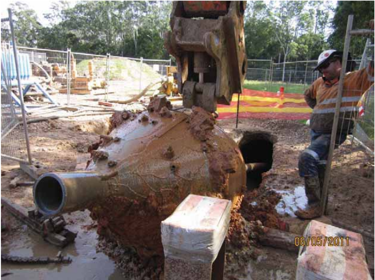
HDD, 54" reamer completed ready for the final 60" reamer before the placement of the pipe. (Work Package 7)
