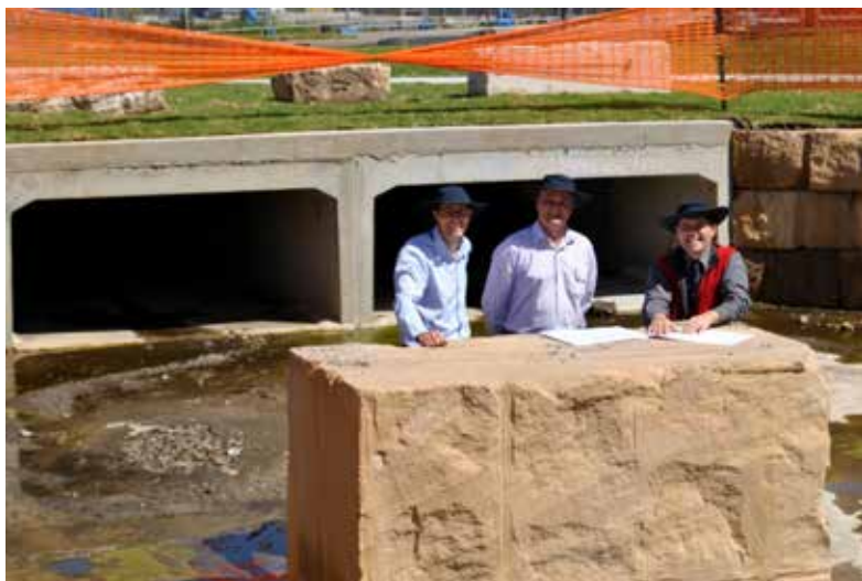
The new drains are 3.6m compared with 90cm drains that were no match for heavy rainfall
