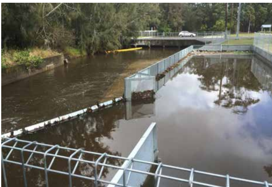
The Long Jetty gross pollutant trap in action
