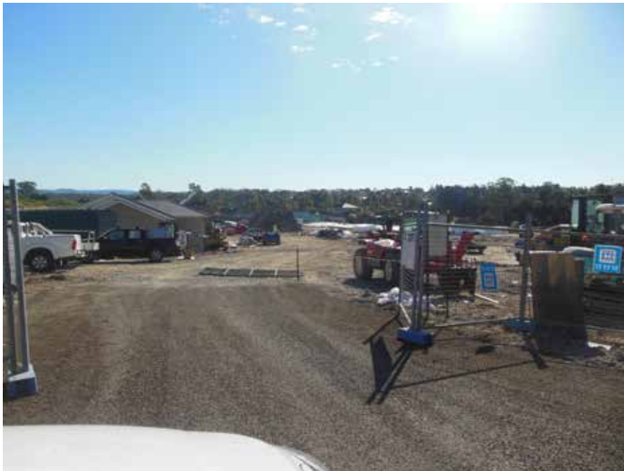
Wyong Shire was appointed as the Principal Certifying Authority on a 67 new dwellings at Hamlyn Terrace
