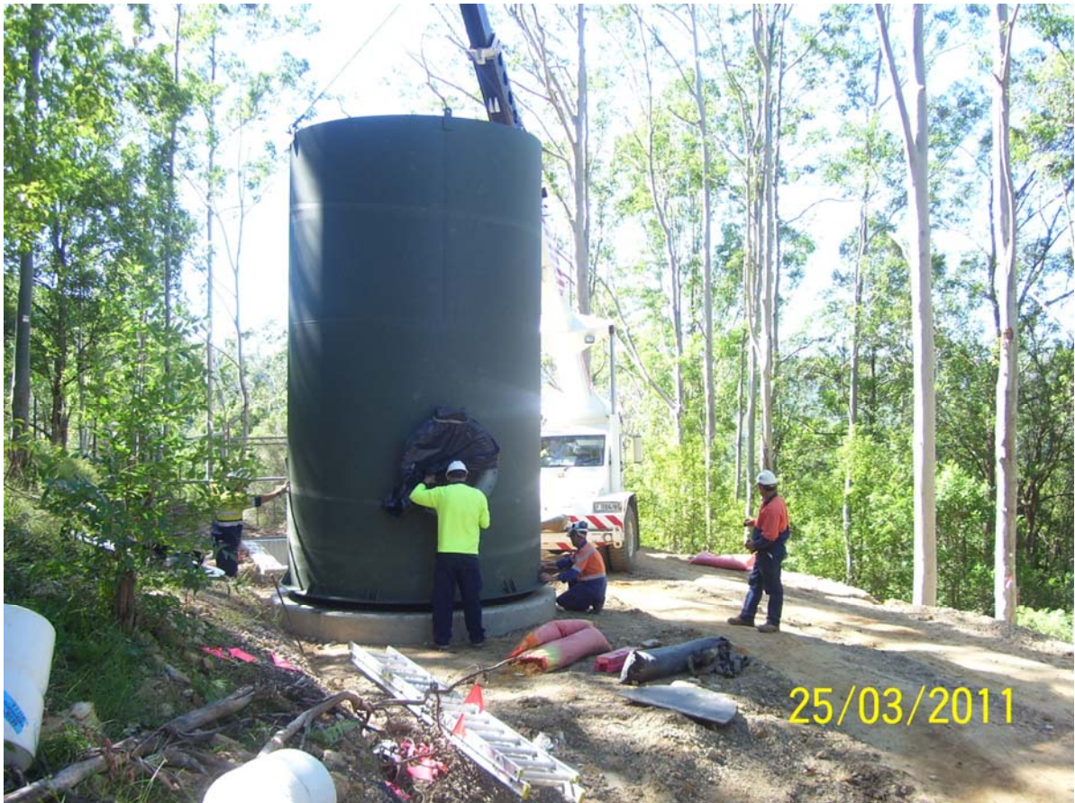
Surge Tank on Mardi to Mangrove Transfer Main being lifted into position. (Work Package 7)
