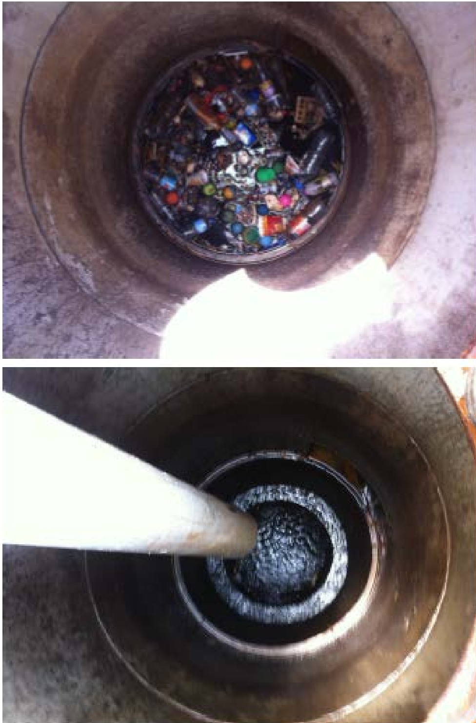
Figure 4: Before and after cleaning photos of an enclosed GPT at Blue Haven
