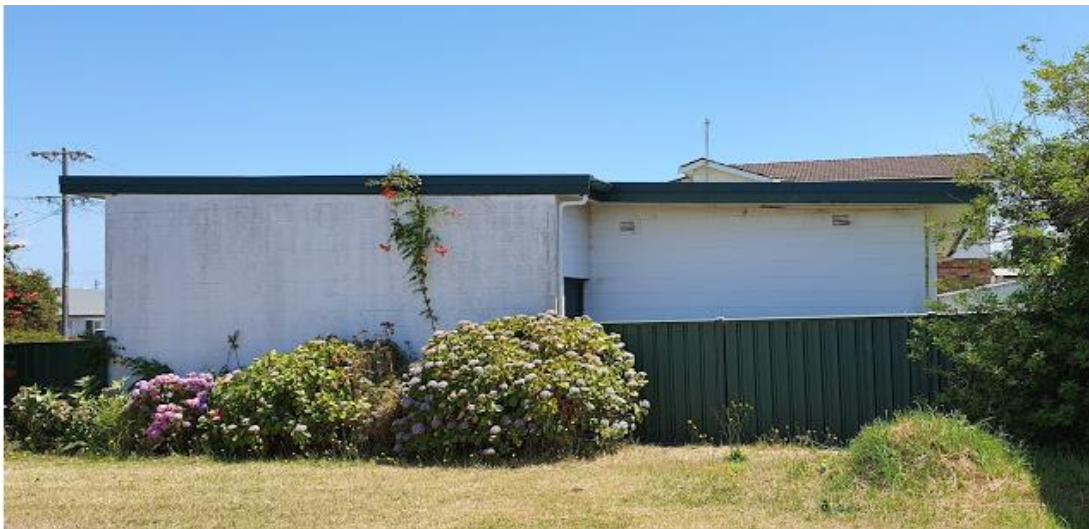
Figure 10 – Photo of external wall of No. 2C Lindsay Street which faces the subject site
