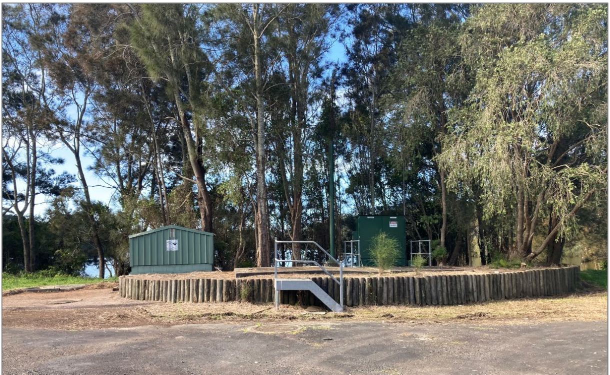
Figure 5 – Sewer Pump Station at northern boundary, facing north
