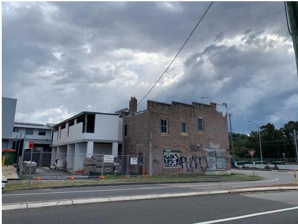
Figure 3 – Rear of development under construction viewed from access driveway at Charlton Street
